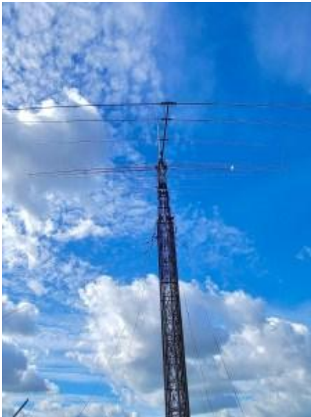
Temporary antenna installed at G2EC - Innovantennas XR56C on Versatower P60
